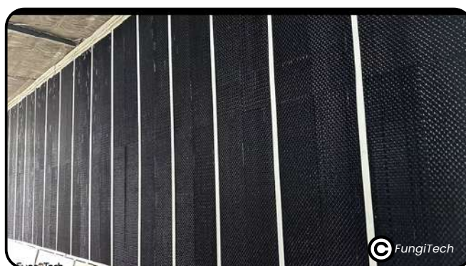
A look at the evaporative cooling system used at Fungitech Sdn. Bhd., designed to optimize growing conditions
